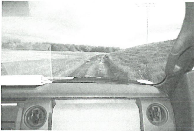
Photo 11: West slope of Pond C, looking north. Note seepage on the intermediate roadway.
