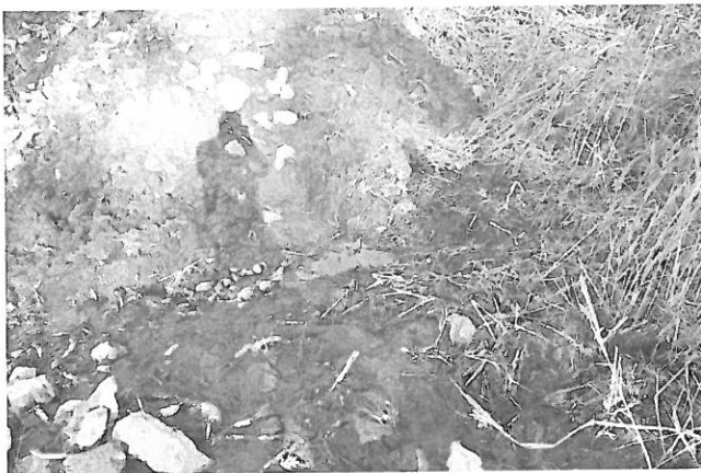
Photo 15: Flow in the ditch along the East perimeter dike of Pond C.
