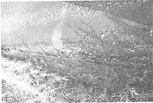
Photo 14: Close up of seepage showing white discoloration.
