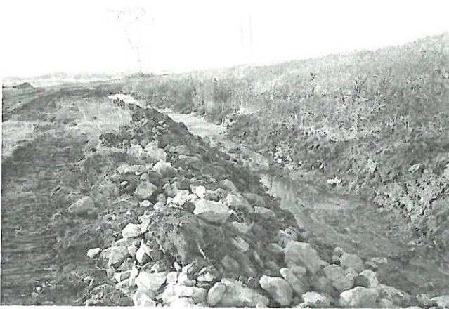
Photo 17: Excavation of the perimeter ditch along the East perimeter dike of Pond C, looking south.
